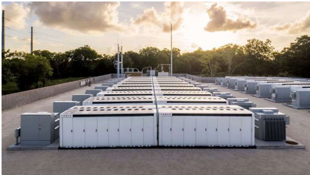
Megapacks installed at a utility site. Source: Tesla
